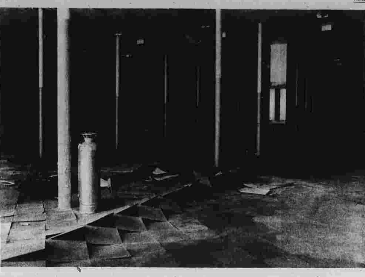
This interior view of the former W.T. Grant store at 811-821 Main St. shows what town officials and area businessmen have termed a horrible and unhealthy situation — floors buckling, ceiling tiles falling off, and ap-
